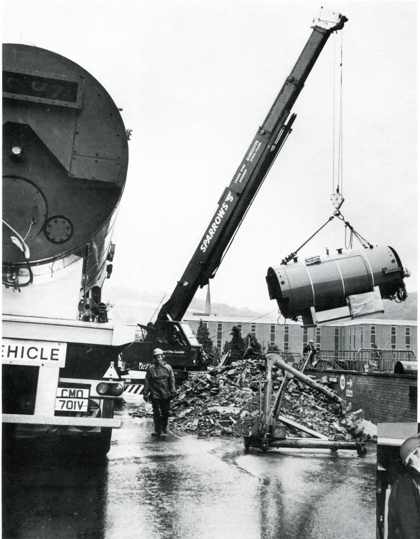
The first of the three shiny red boilers swings slowly across and hovers over boiler house no.2. Several dummy runs were necessary and the rain made a tricky operation even trickier.
